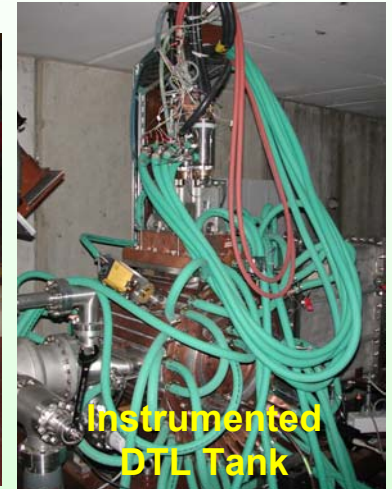
IFMIF DTL Tank (CEA Saclay)
